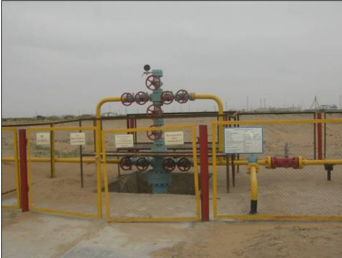
Figure A.1: Surgil Field Wellhead
