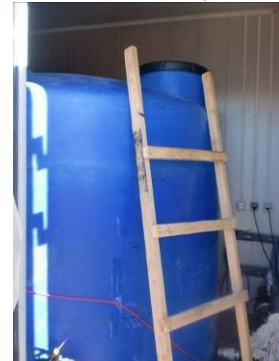
Figure A.10: Potable Water Storage
