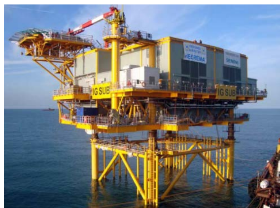
Typical offshore collector platform
